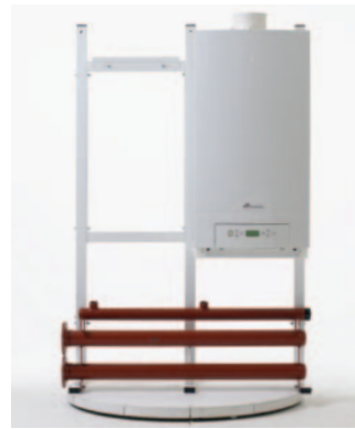
Step 3 Individual GB162 V2 boilers are mounted securely on the framework.
